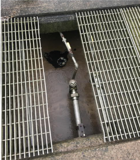
Surface Foam Drains through Pipe to Aeration
