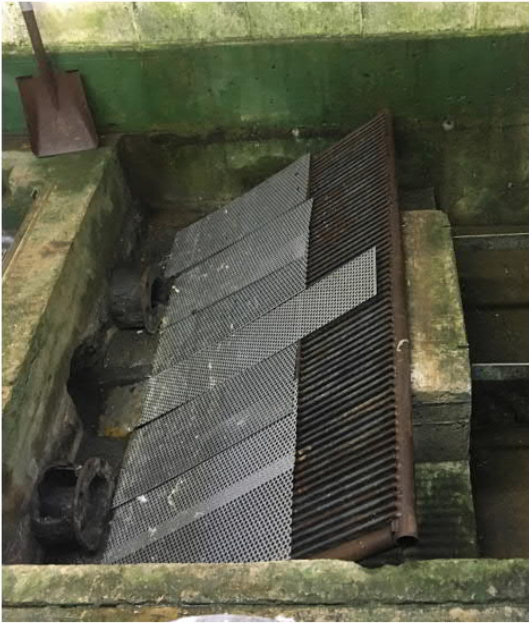
Headwork Screening Infrastructure
