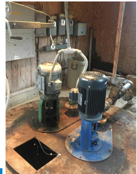
Effluent Pump Station
