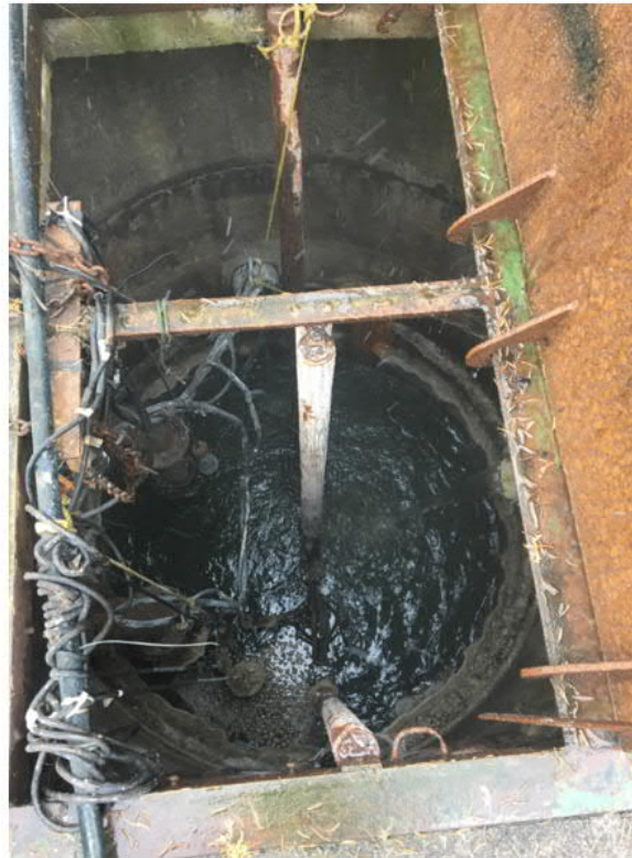
Influent Pump Station
