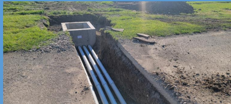
(TOP) INTERSECTION EXCAVATION (BOTTOM) PULL BOX AND DUCT BANK AT TAXIWAY A4
